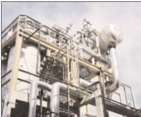
Process Dynamics hydrocracker at Giant Industries refinery in Gallup, N.M.
